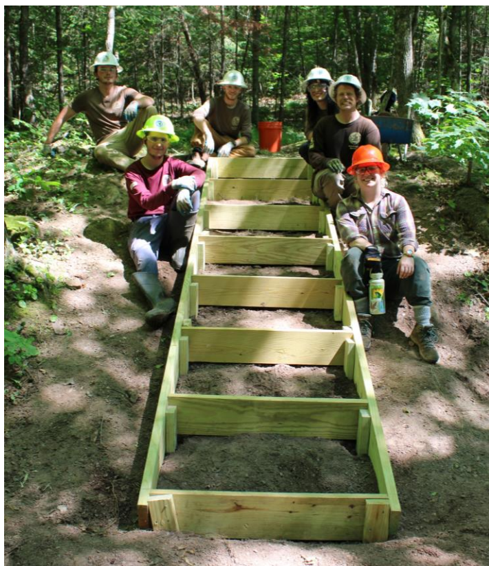
The crew is proud of the steps they built on a steep slope near Esox Lake. L – R: ACE members Conor Lackner, Walker Hoskins, Ryan Winter, Cassidy Ivey, Elijah Gabel, and USFS staff Kaelin Hall.
