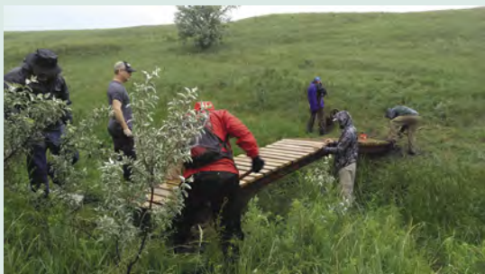
Volunteers install one of two 25-foot boardwalks in pouring rain at Lake Ashtabula.
